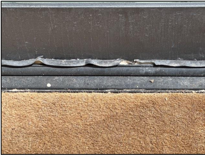
Weatherstripping missing or ineffective
