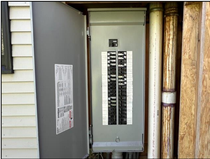
Breakers - exterior wall
