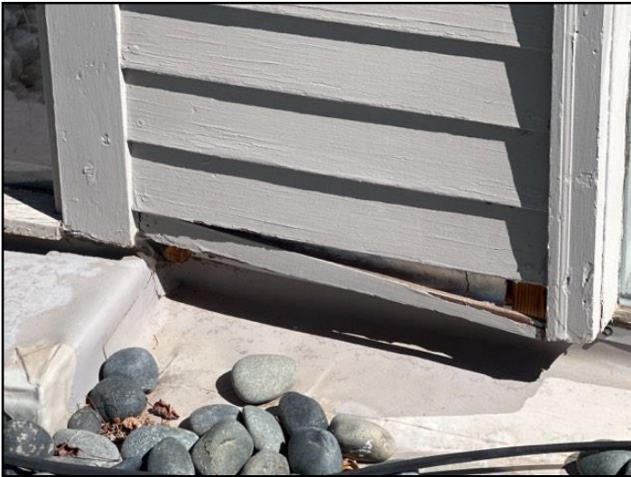
Cracked, split or broken
