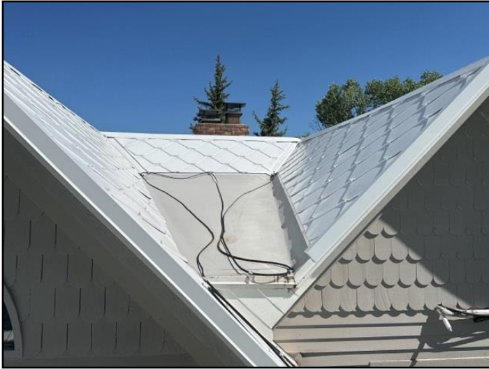
Vulnerable to ice damming
