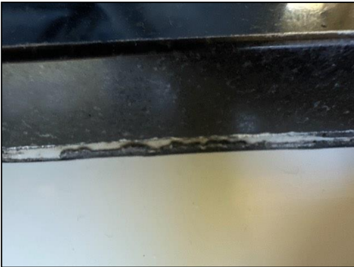
Caulking loose, missing or deteriorated
