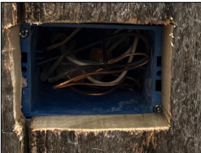
Damaged, loose or missing
