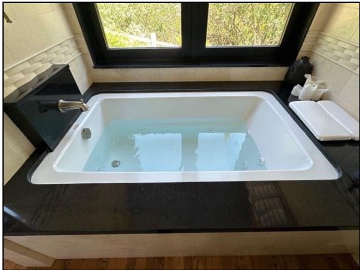
Caulking loose, missing or deteriorated
