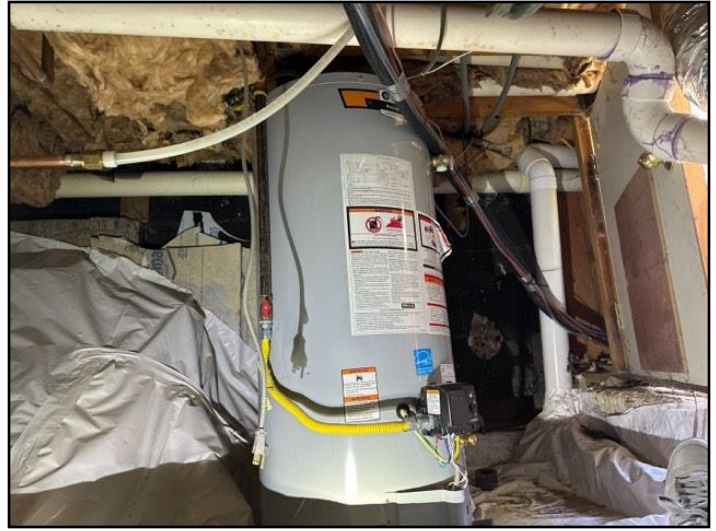
No drip leg (sediment trap, dirt pocket)
