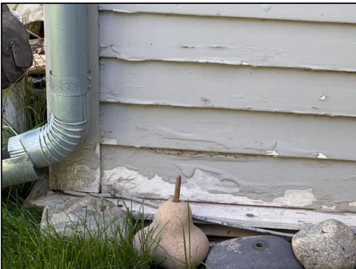
Paint or stain - needed
