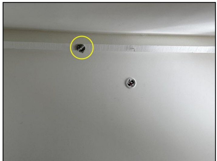
Damaged, loose or missing
