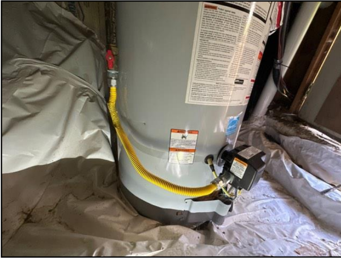
No drip leg (sediment trap, dirt pocket)
