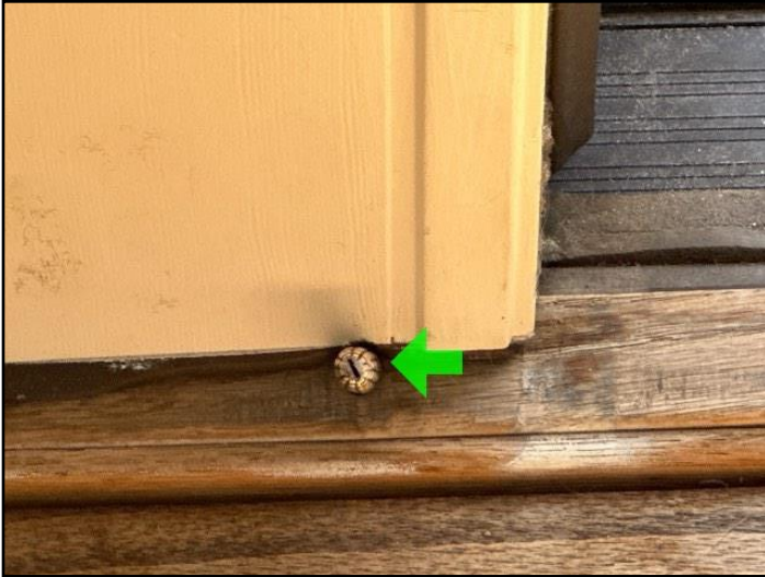
Missing or damaged
