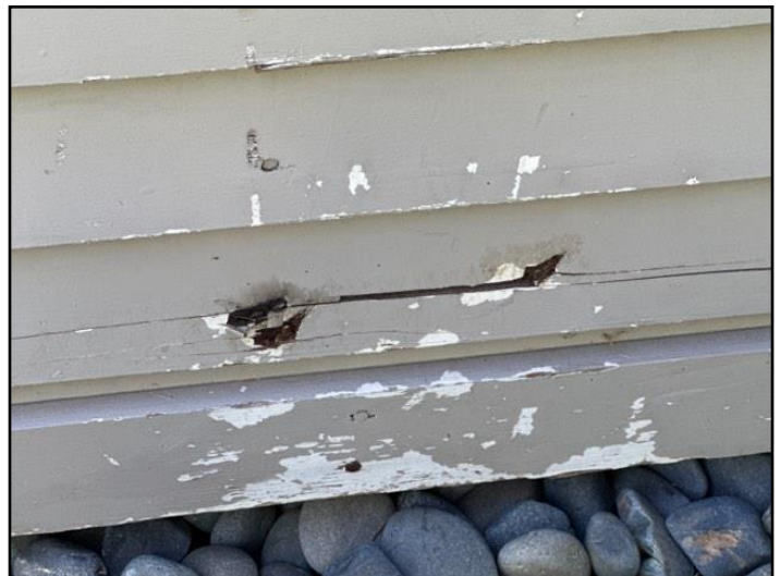
Paint or stain - needed
