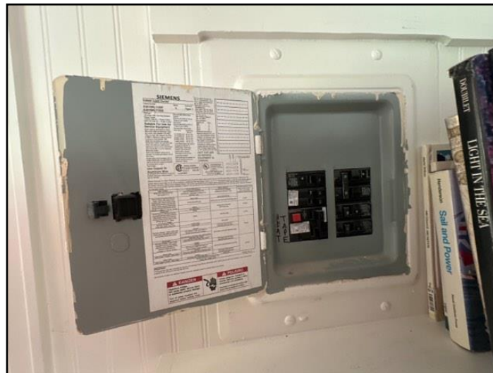
Breakers - first floor
