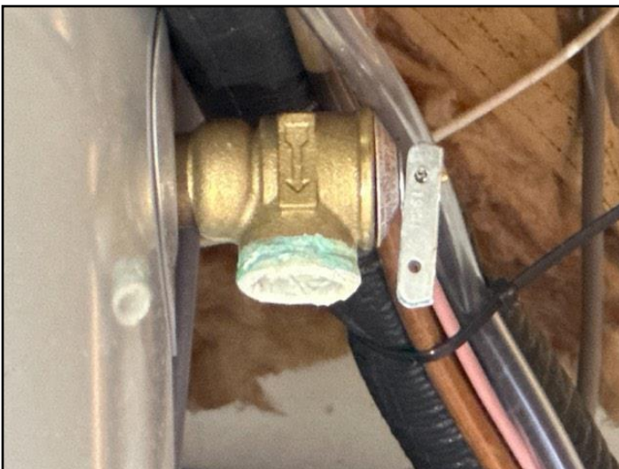
Discharge tube missing
