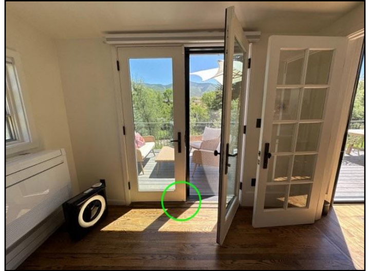
Missing or damaged
