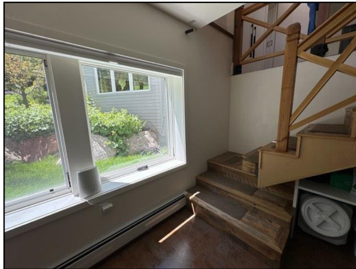
Safety glass not installed
