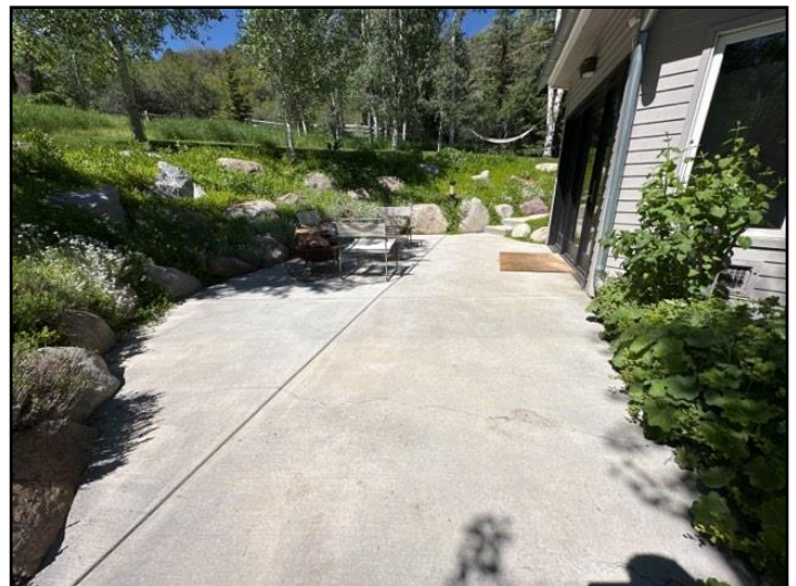
Cracked or damaged surfaces
