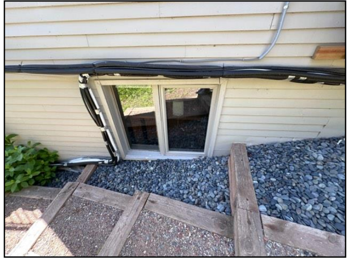
Inadequate sill projection
