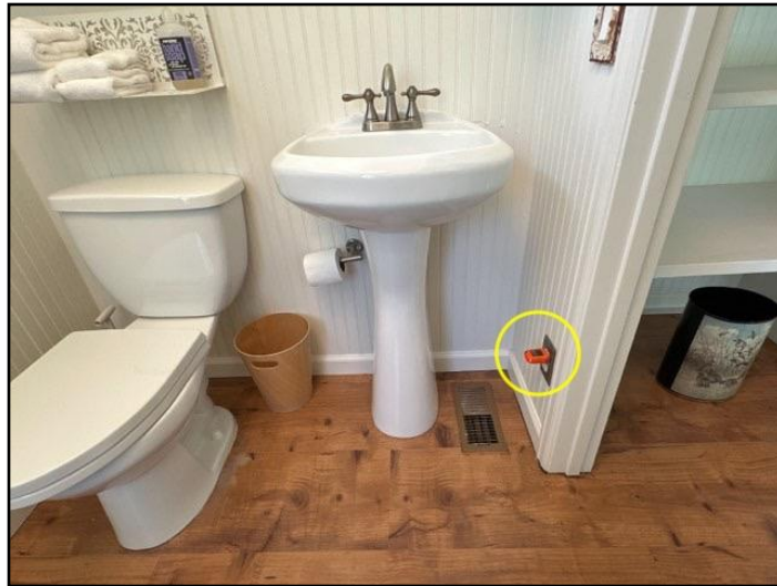
GFCI/GFI needed (Ground Fault Circuit...
