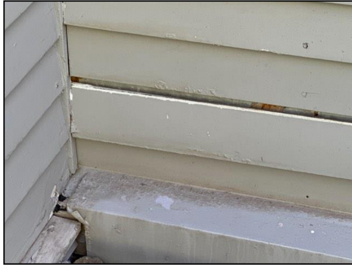
Cracked, split or broken
