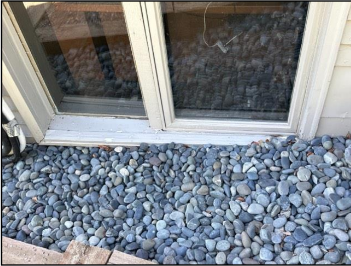
Inadequate sill projection
