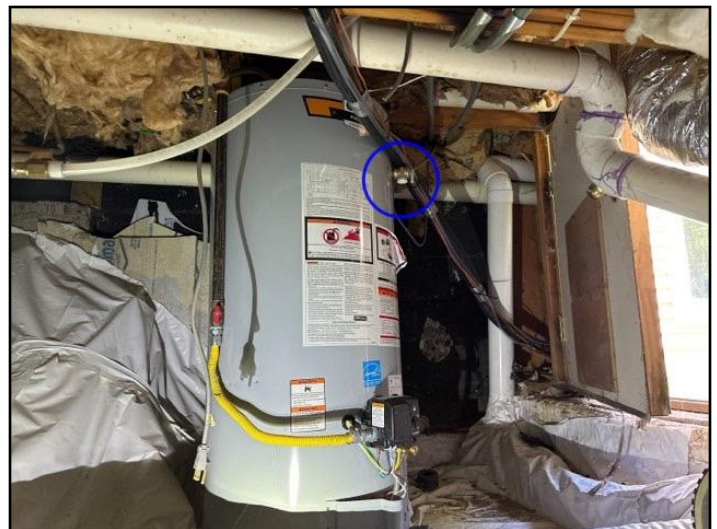
Discharge tube missing
