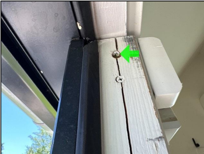
Missing or damaged
