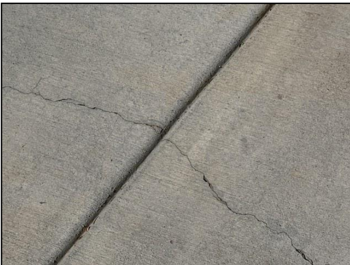
Cracked or damaged surfaces
