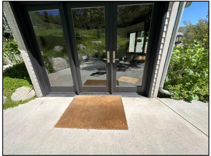
Weatherstripping missing or ineffective
